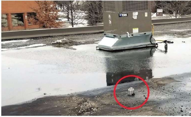
An example of a basic roof drainage system, featuring a roof drain connected to interior drainage piping, critical for preventing water accumulation on flat surfaces.
