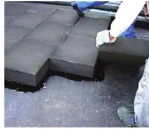
Installing insulation on a concrete roof deck using a compatible adhesive, adhering to best practice guidelines for secure material placement.
